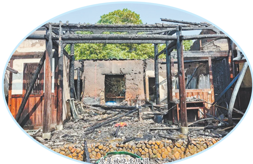
房屋被烧空坍塌
